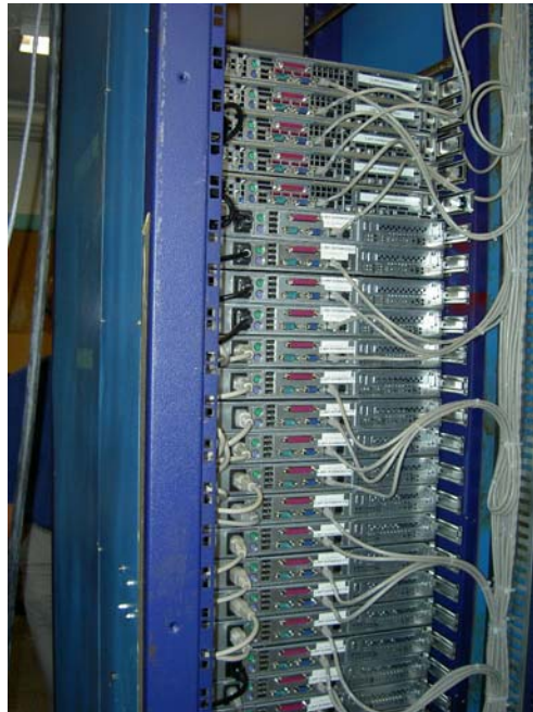
Figure 3: cabling of the PCs in the rack.
